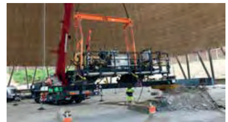
It took about 14 hours to lift the robot and equipment the 162m to the top of the 162m chimney.
